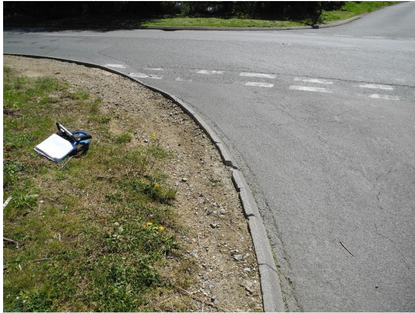
Image 4 – Whitehouse Road – verge overrun on eastern side of road
